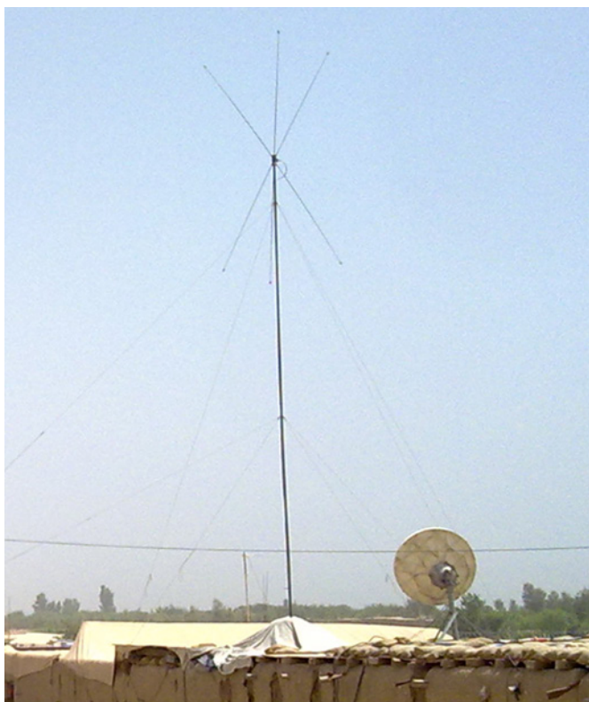
Semi-static MPT-1327 BSN mast/antenna at sub-tropical location
